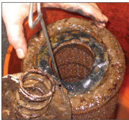
Image 4: Filter with evidence of corrosion deposits (due to its brown colour). It is completely plugged with bio-film and corrosion particles.
